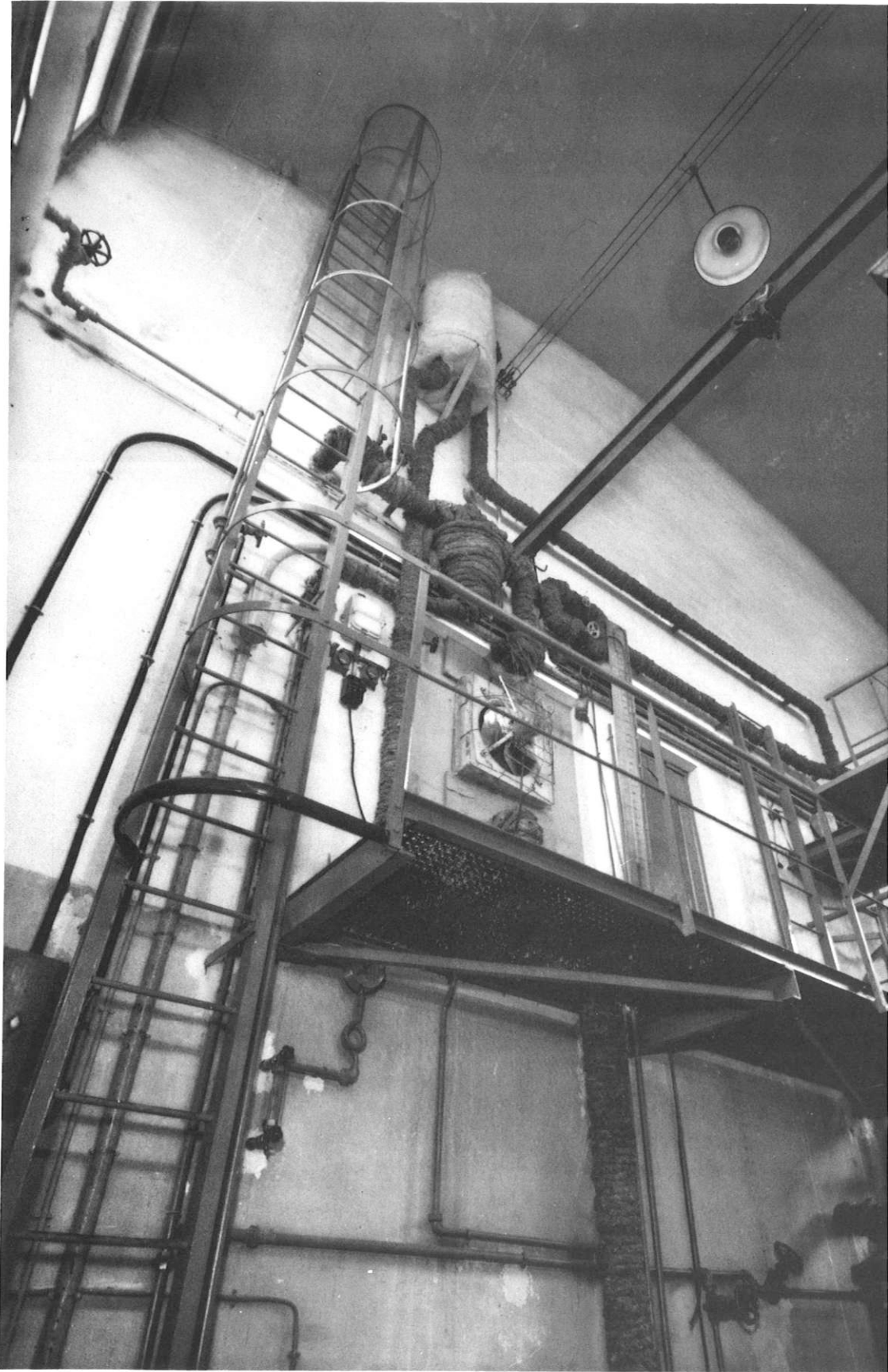
UNIT HEATER TEST STATION
