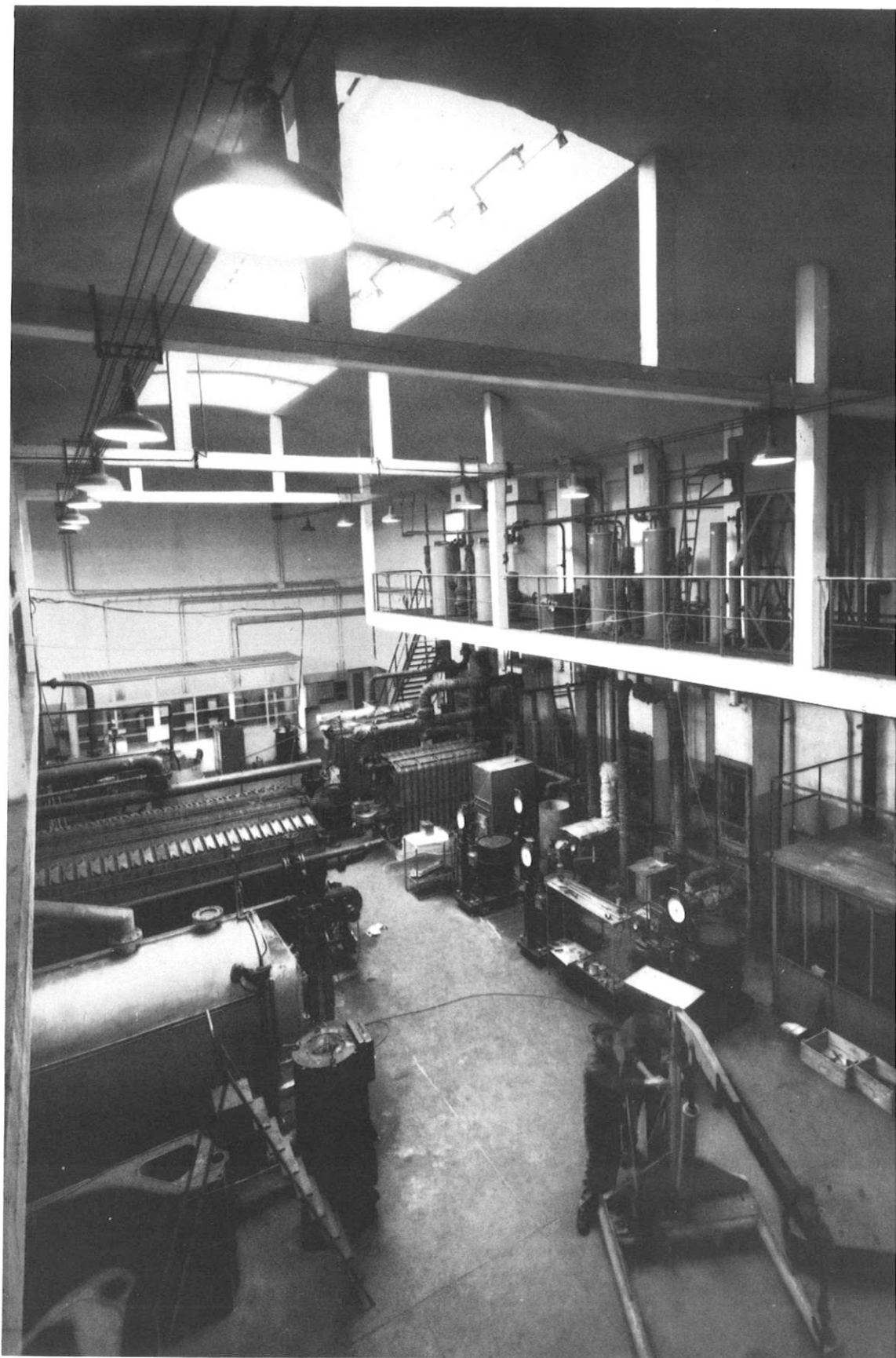
GENERAL VIEW OF BOILER TESTING ROOM
