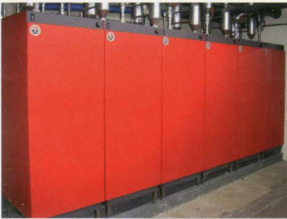
An ACV cascade of six boilers
